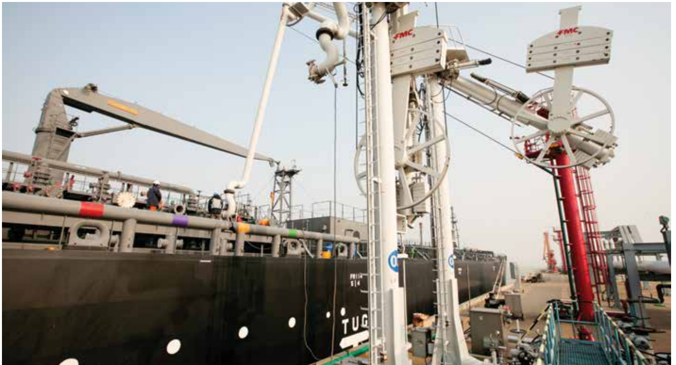
Jet fuel discharging from vessel at port
