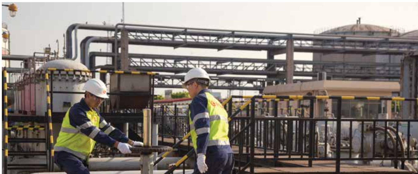
Handling of oil storage tank valves 开储油罐阀门
